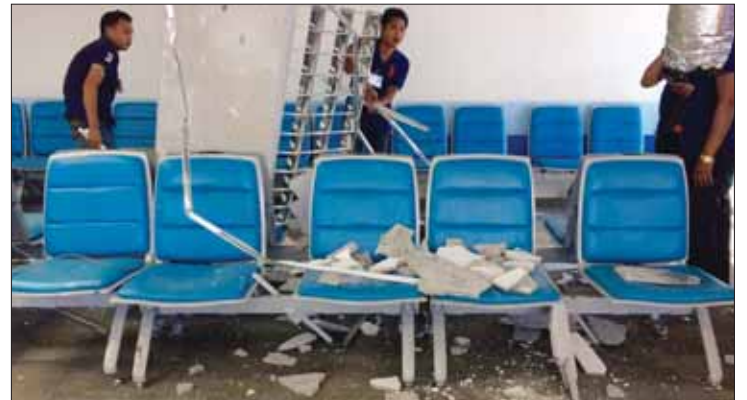
The falling ceiling injured one passenger. Photo: Kritsada Mueanhawong
