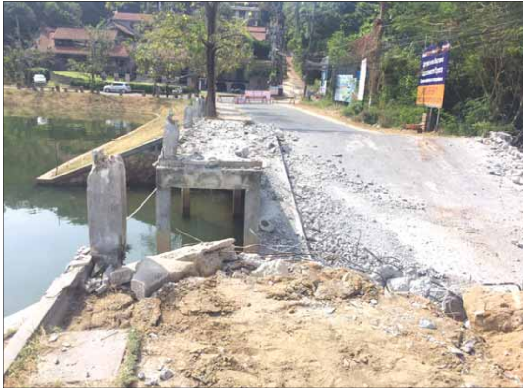
The bridge on the road around the Nai Harn lake in the area of Naiharn Beach collapsed earlier this week. It is now under construction, with the budget of 1.3 million baht, by Rawai Municipality. The project is expected to be completed in 2-3 months. During this time, authorities have asked commuters to use the diversion instead, signs for which were placed at the site in English and in Thai. Photo: Rawai Municipality
