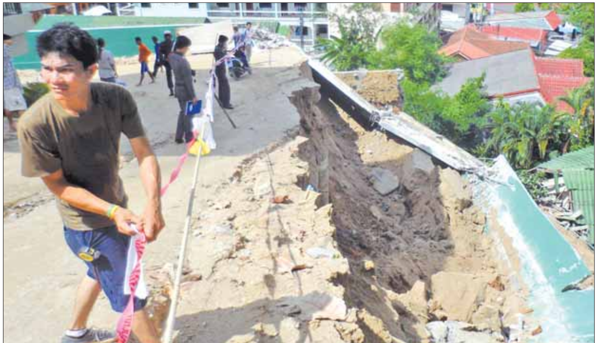
The view from the resort in Patong showing the collapsed wall which fell onto houses below.
