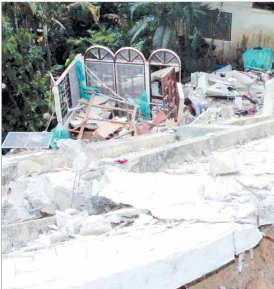
The house below the collapsed wall has already been demolished by workers who will build a new home paid for by the hotel owner. Photo: Kritsada Mueanhawong
