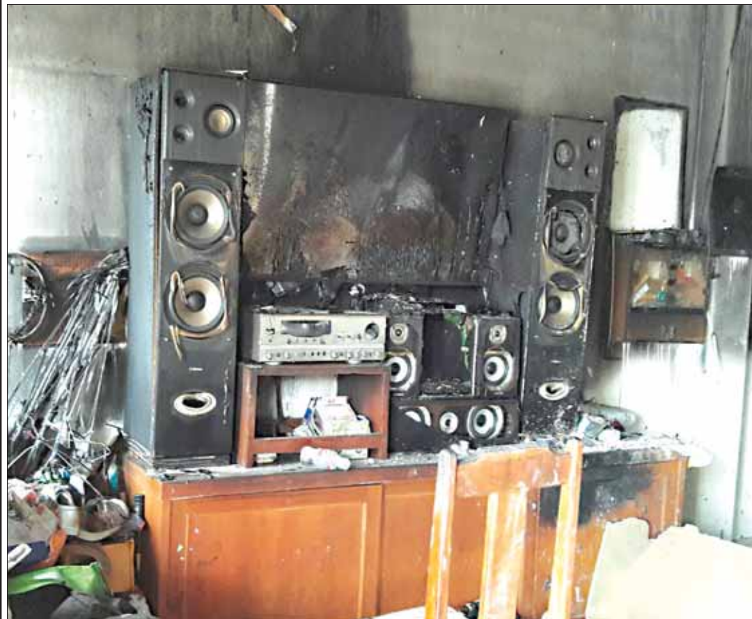
A fire gutted a house in Phuket Town on the morning of October 31, which left the owner, Suthi Angsithakun with about 200,000 baht worth of damages. Firefighters took over 20 minutes to put out the blaze before it spread to nearby houses. The cause of the fire was still unknown at press time. Photo: Kritsada Mueanhawong
