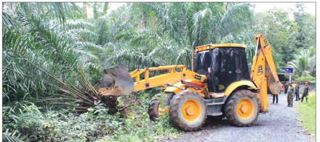
Heavy machinery was brought in to demolish plantations said to be encroaching on public land in Thalang. Photo: Kritsada Mueanhawong.
