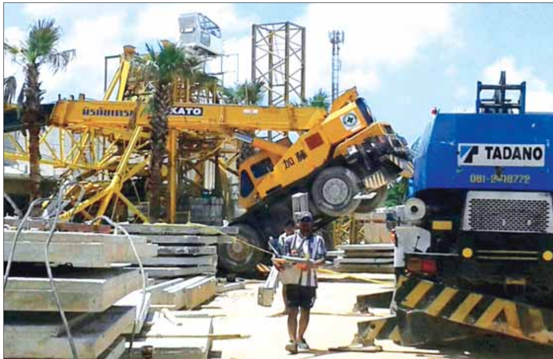
Police have ordered a halt to construction of an eight-storey building near Phuket International Airport, after a crane collapsed at the site on June 10, killing one construction worker and injuring three others. The cause of the crane collapse is still unclear. Kritsana Crane Company and the developer, Phuket Sirinath Property, have been ordered to stop construction while investigations are underway. The injured were taken to Vachira Phuket Hospital. Photo: Kritsada Mueanhawong
