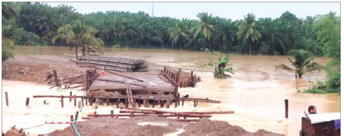
Motorists are advised to use Petchkasem Road after temporary alternative route collapsed. Photo: Pornthip Paklao, Ao Luek Municipality
