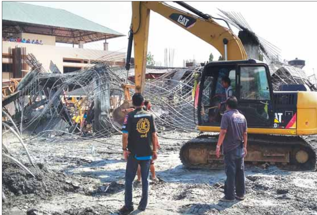
Police announced that they will press charges against the construction company involved in a building collapse that killed five female workers at the Institute of Physical Education's Krabi Campus in March. Sections of unhardened cement fell on the women working on the floor below. Police said the rebar used did not meet the legal requirements of construction materials, and there was no qualified engineer on site at the time. Photo: Kritsada Mueanhawong
