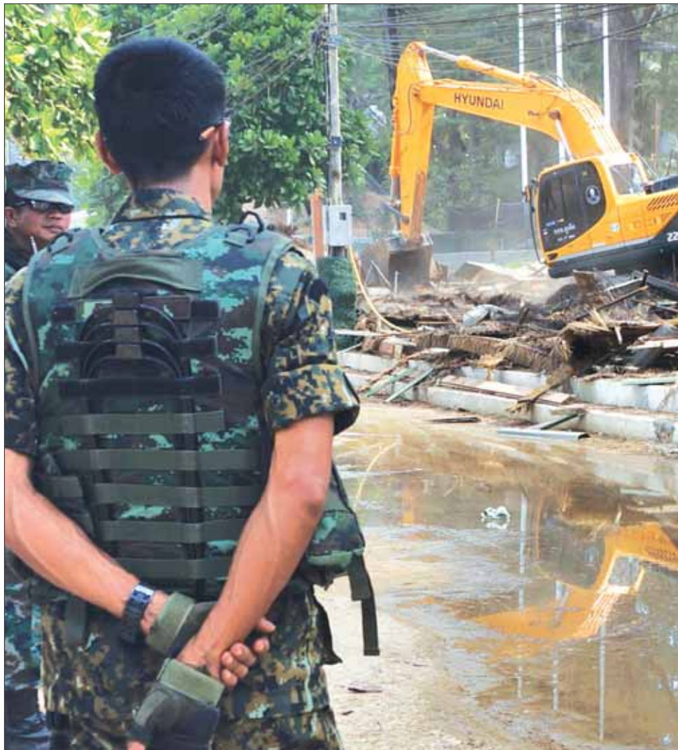
Military personnel were on site as the demolition began. Photo: Chutharat Plerin
