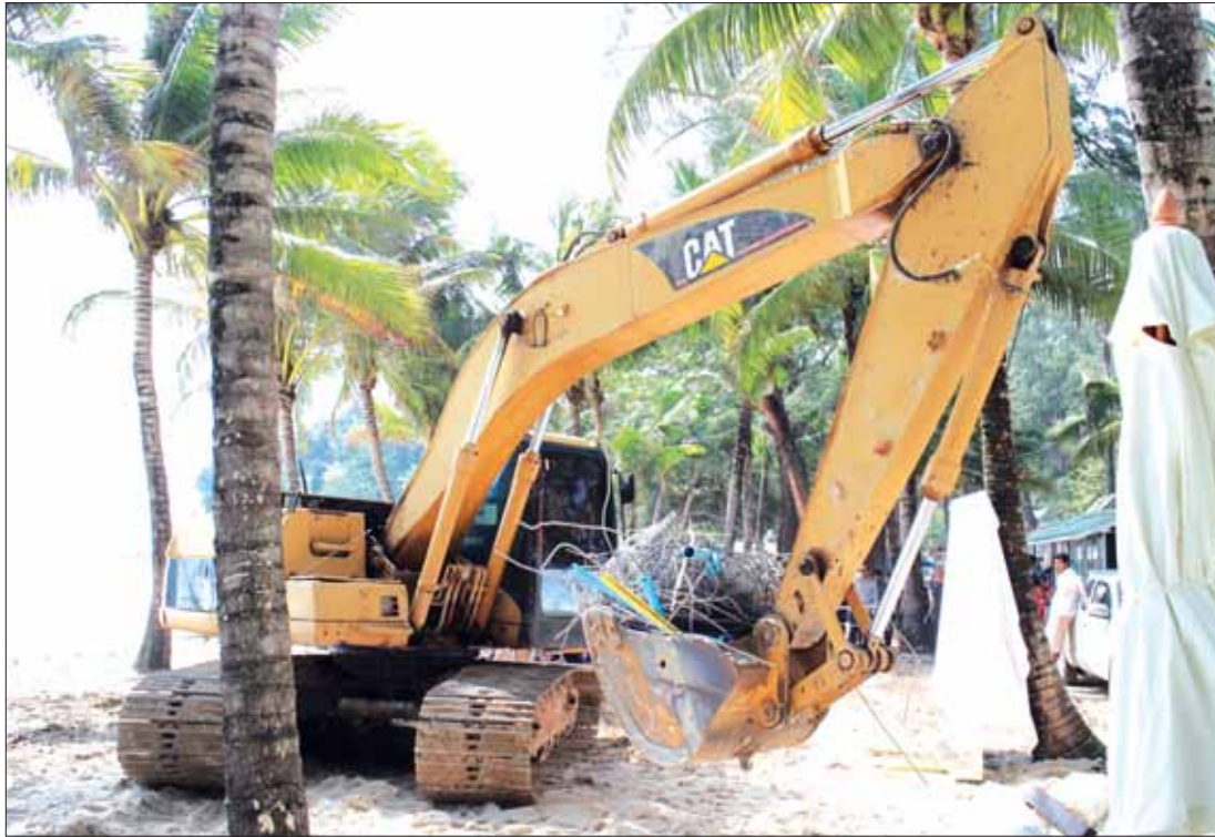
Vice Governor Chokdee announced the imminent demolition of illegal businesses at Surin, Lay Pang and Layan Beach. Photo: Gazette file
